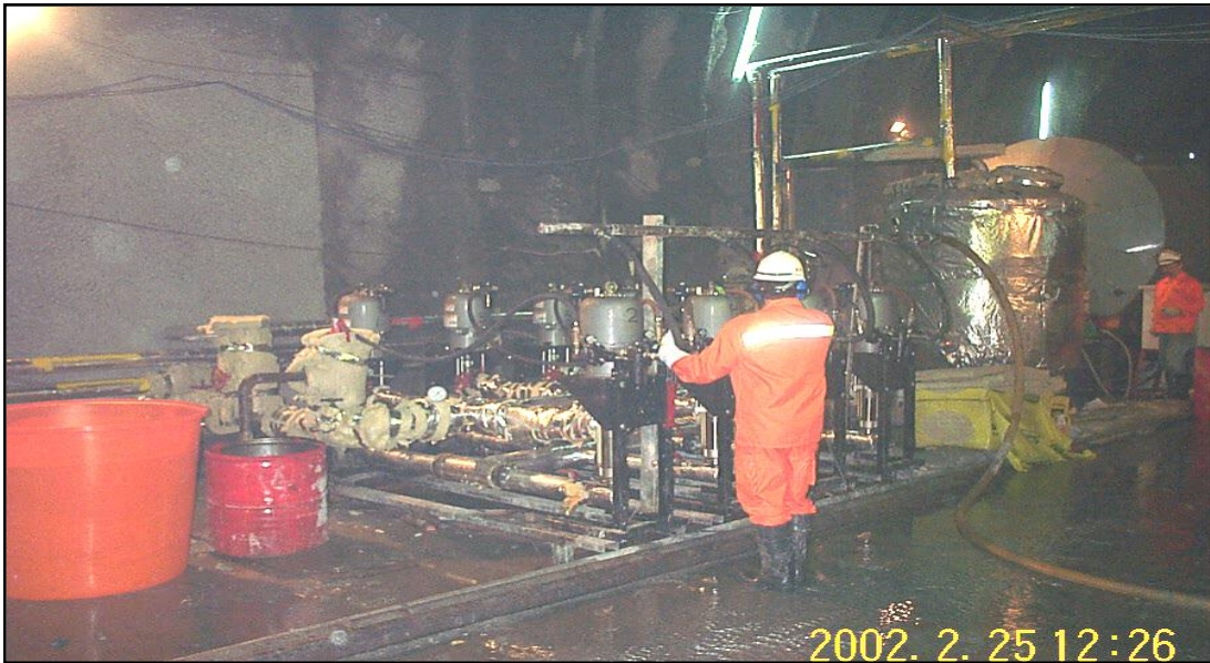
Figure 5: Grout plant in foreground, insulated bitumen holding tank in background
