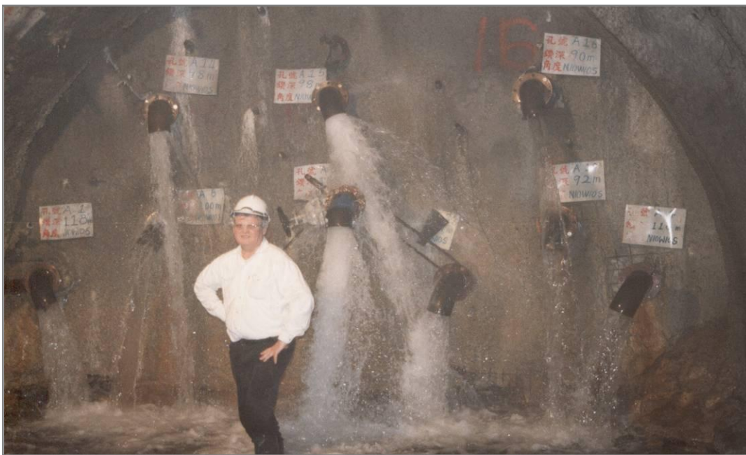
Figure 1: View of Drainage Tunnel with 36 pressure relief pipes
