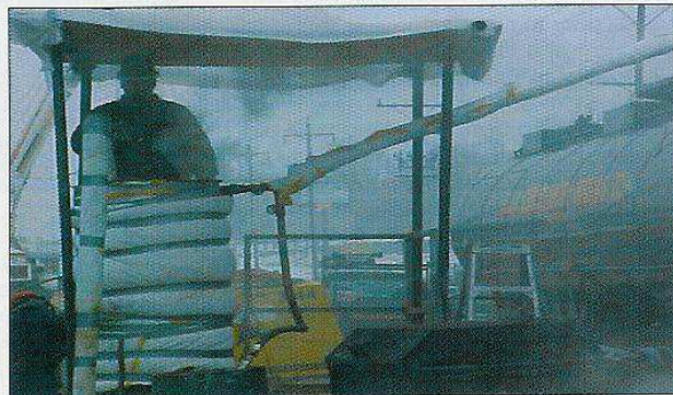
Figure 15 Hot bitumen transfer station
