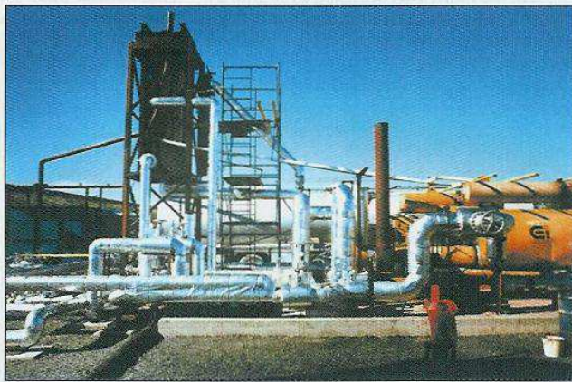
Figure 10 Custom built hot bitumen plant
