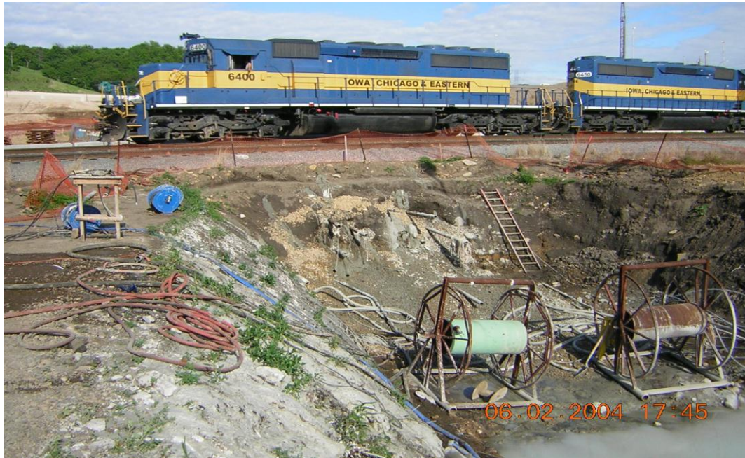
Photograph 1: Sleeve pipes installed through the CP railway embankment around the planned tunnel trajectory
