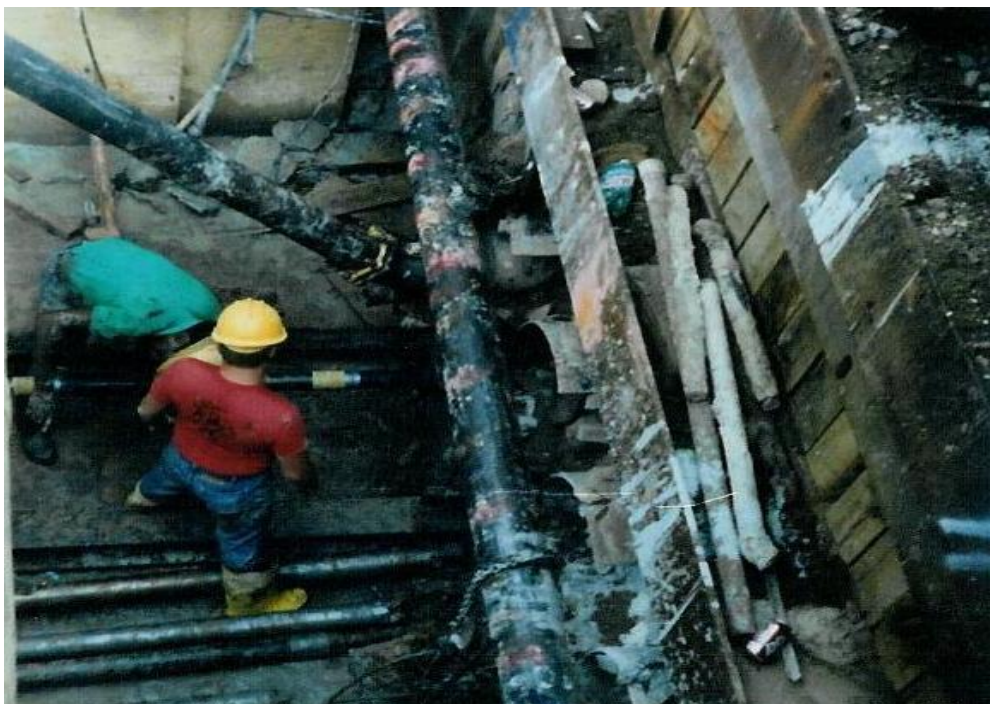
Photograph 5: Grouting crew during the installation of one of the steel sleeve pipes
