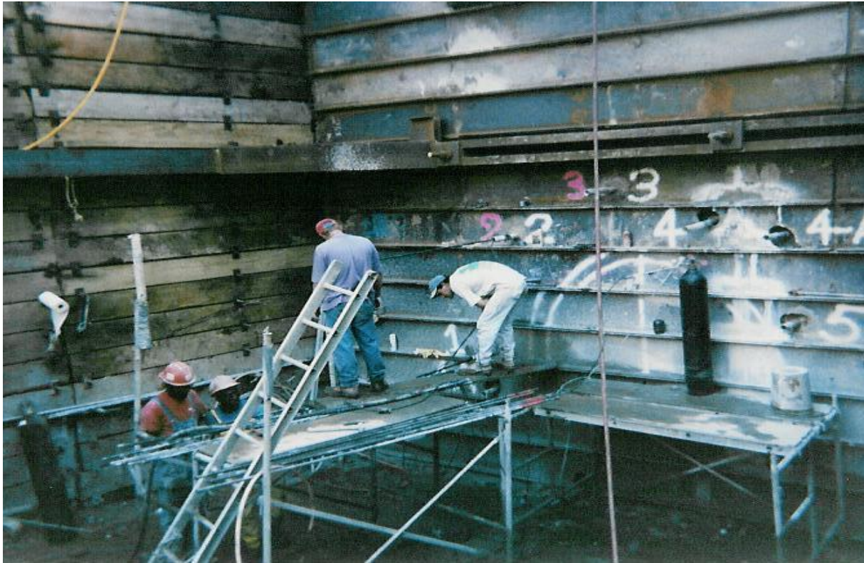
Photograph 4: Grouting crew performing injection of sodium silicate based grout via the sleeve pipes
